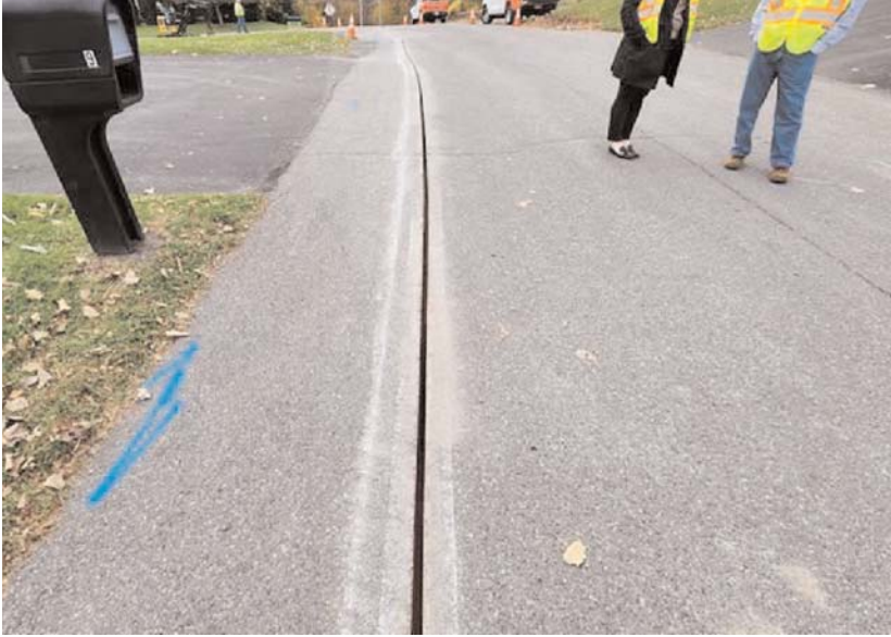
This "microtrench" was being installed by Archtop Fiber earlier this month on a residential street in Saugerties. The trench is then covered over, sealing the cabling inside.
