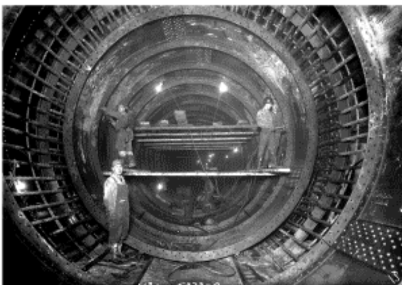
Bolting together the reinforced steel lining prior to concreting the Delaware Aqueduct, 1942. Photo courtesy of the NYC DEP Archives.
