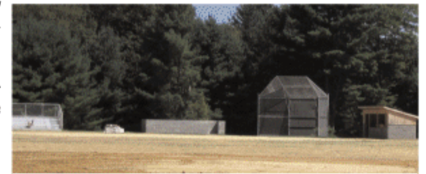
The new dugout was built by TVCS students in Mr. Pompeii's and Mr. Huebsch's class on the baseball/soccer fields that are under construction.
